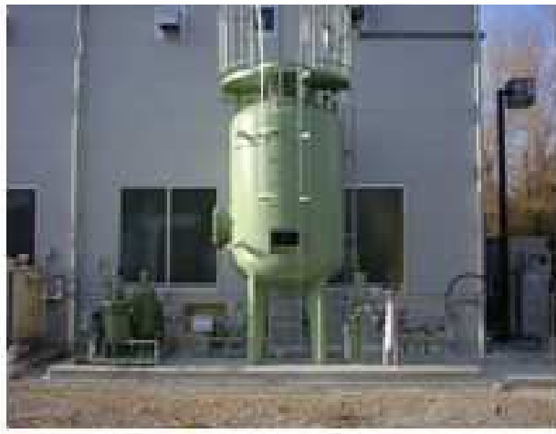
Figure 10. The adsorptive biogas storage system
