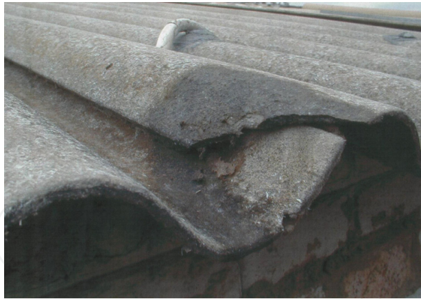
Figure 3. Detail of asbestos roof sheet in Soweto, showing damage and exposed asbestos fibres. (Courtesy of Professor JI Phillips).
