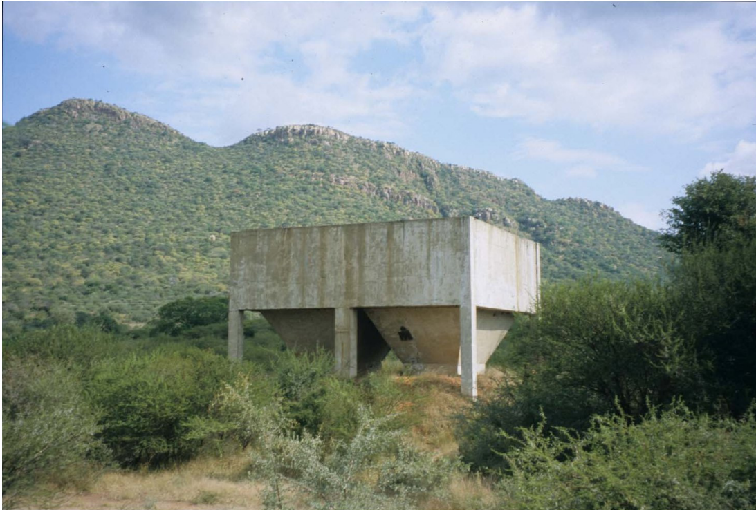
Figure 7. Derelict ore bins at Penge mine. (Courtesy of Dr Koichi Honma).
