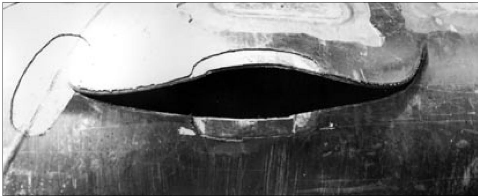
Figure 17. Burst initiated on slit B – a detail
