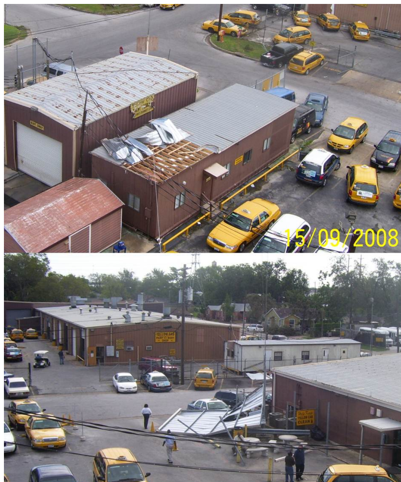
Figure 12. Structural damage caused by Ike as viewed from the tower at approx. 18 magl towards NE (top) and ESE (bottom)
