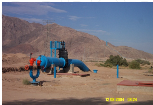
Figure 7. Valve system of a desert water aqueduct.
