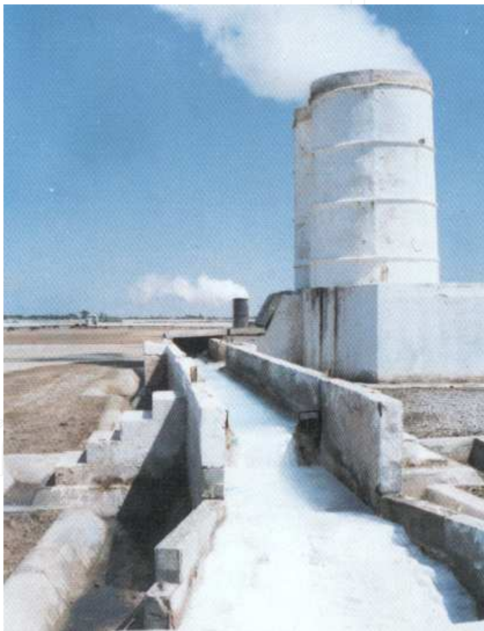
Figure 15. Corrosion in concrete structures used to separate steam from water and to operate steam silencers.
