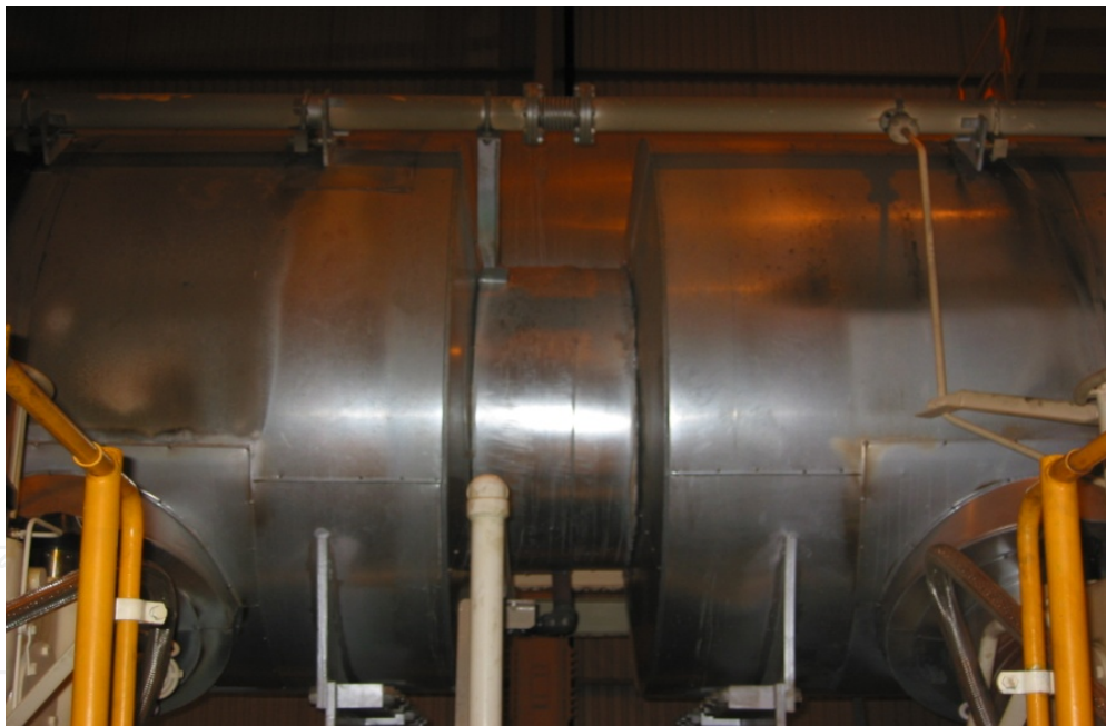
Figure 14. Stress corrosion cracking, in a combustion gases pipe of a thermoelectric station.
