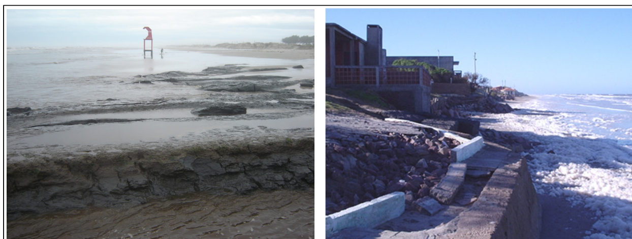
Figure 3. Pictures showing beach erosion indicators. The left picture shows mud outcropping at the beach and the right one the buildings destruction due to sea level rises during storms.
