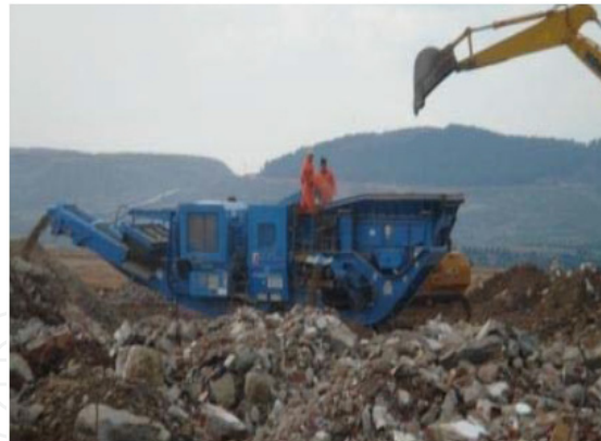
Figure 3. Demolition Waste Recycle Facility [35]
