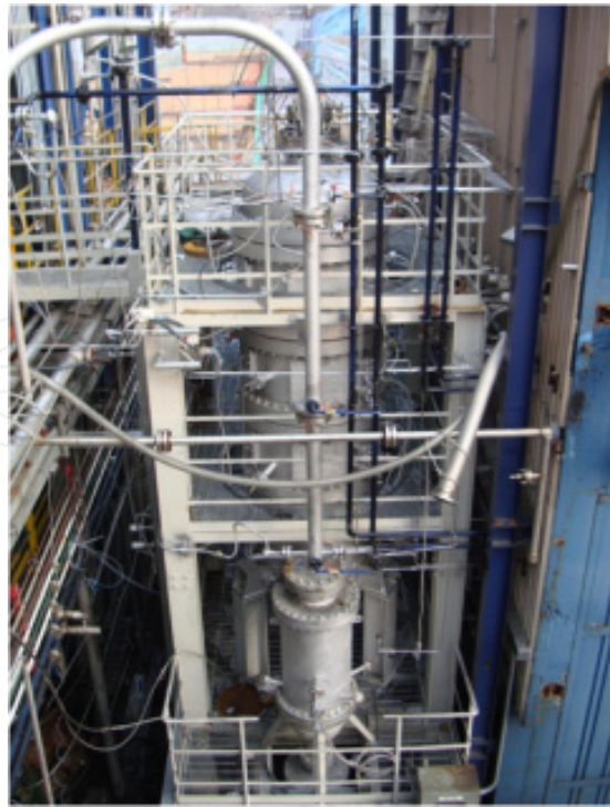
Figure 2. Pilot-scale coal gasifier of top-feeding, partial/non-slugging entrained-bed type (max. 21 bar)
