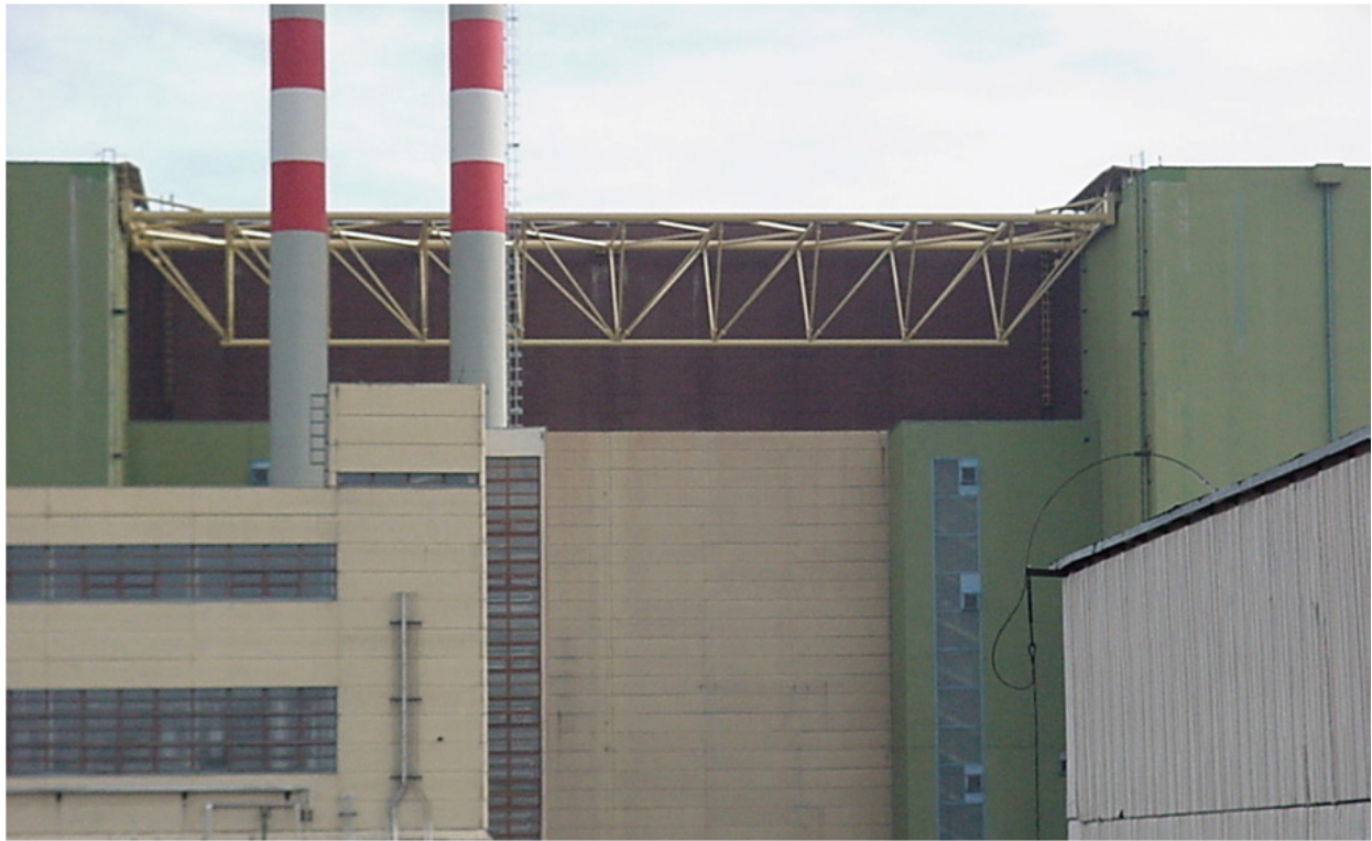
Figure 3. Steel-frame bridge between localisation towers for fixing the frames of the reactor hall (columns) in cross-wise direction
