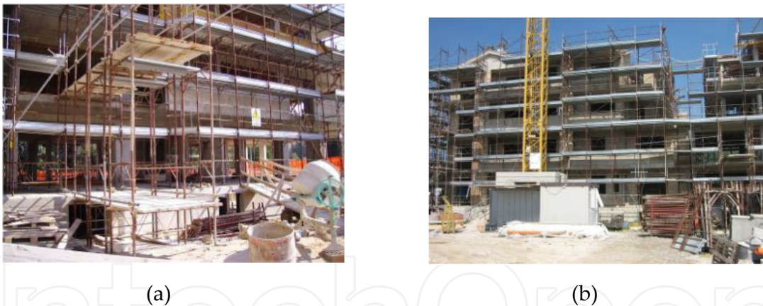
Figure 5. Typical conditions of a construction site in an advanced construction phase, (a) just after the structural frame completion and (b) after the construction of the envelope and of the internal partitions.
