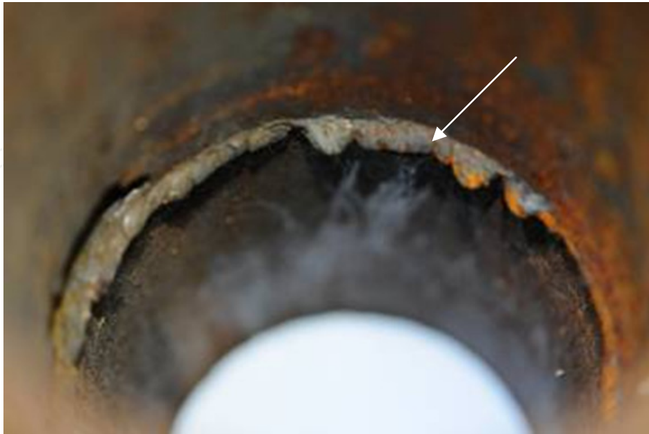
Figure 14. The inner side of circle area in Fig. 11 showing an excessive overfill (arrow) in the failed pipe at 12 o'clock position.
