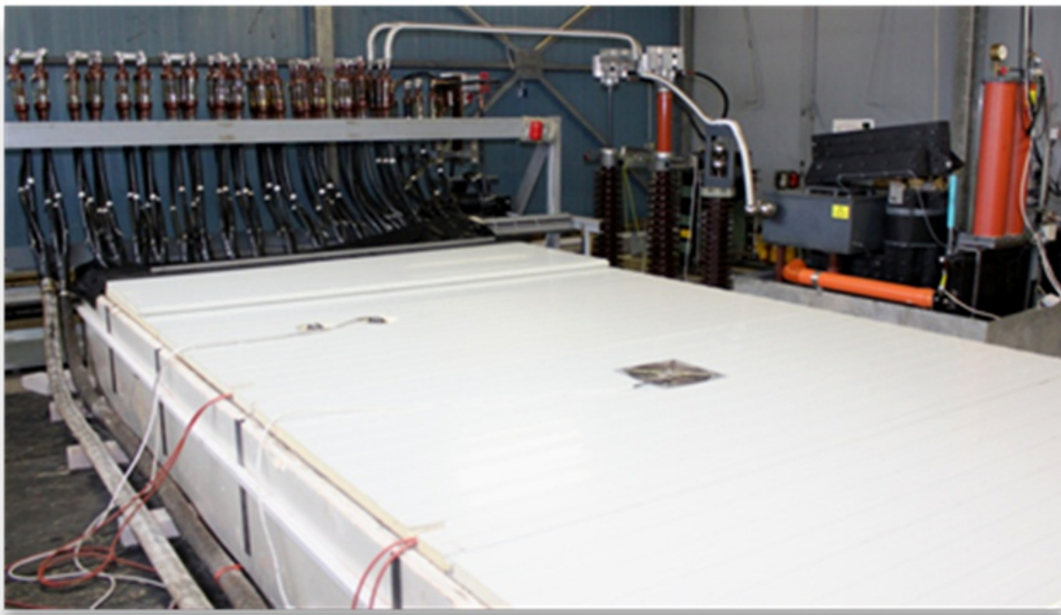
Figure 11. Partial overview over central components of the ICAAS system (transformers for voltage and current generation, overvoltage protection, rectifiers, etc.) and cable samples
