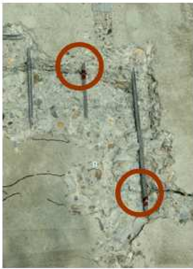
Figure 9. Failure of concrete beam after fatigue loading test.
