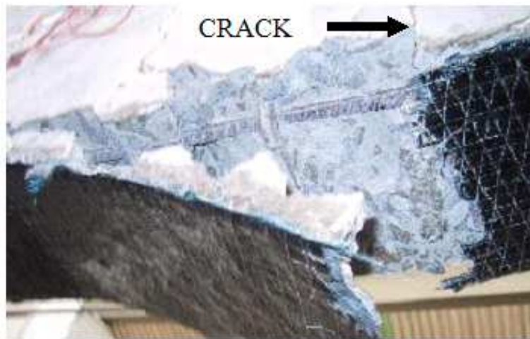
Figure 8. Rupture of FRP close to a flexural crack tip.
