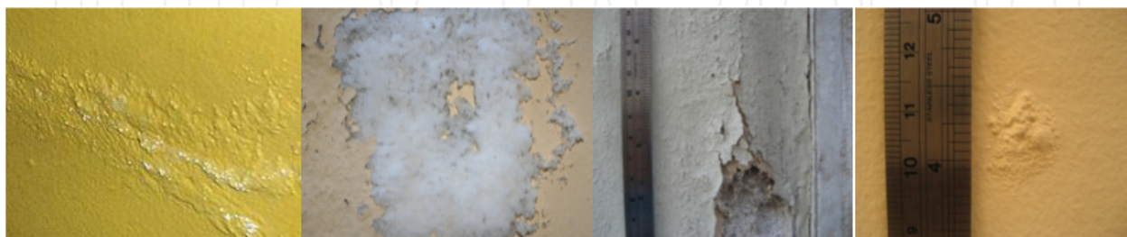
Figure 11. Swelling, efflorescence, cracking and blistering (Moura, 2008).
