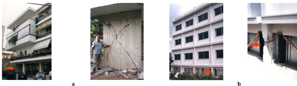
Figure 3. a Typical damage of shear walls at the “soft story” during The Kozani 1995 Earthquake in Greece. b. Typical damage of “short” columns during The Kozani 1995 Earthquake in Greece.
