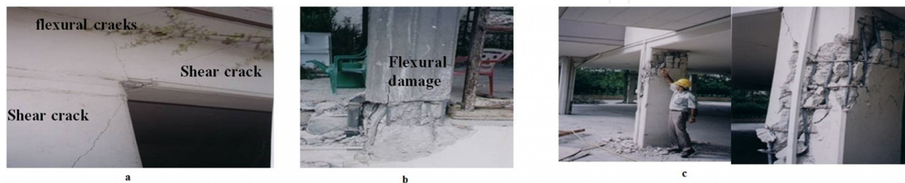
Figure 2. a Typical damage of beam at the joint with the nearby column (6 th story building, Aharnes, Athens earthquake 1995), [2]. b Typical damage of the toe of a column at ground floor (two-story building, Nea Kifisia,, Athens earthquake 1995), [2]. c Typical shear damage at the columns of a “soft story” (4-story Metamorfofi building, Athens earthquake 1995), [2].
