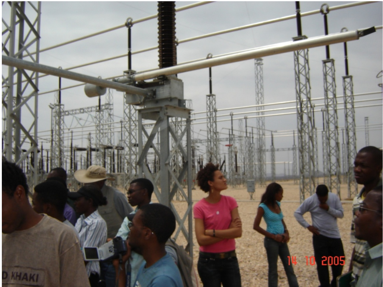
Fig. 3. A group of Polytechnic of Namibia students visit the AUAS 400 kV substation
