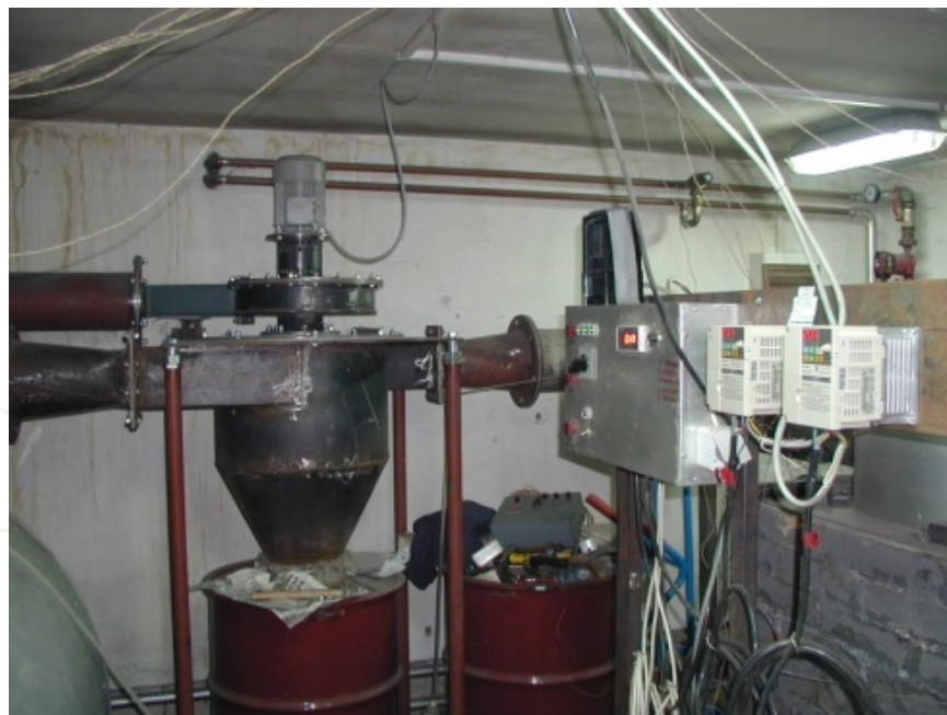
Figure 5. The boiler control system and cyclone-type particle precipitator
