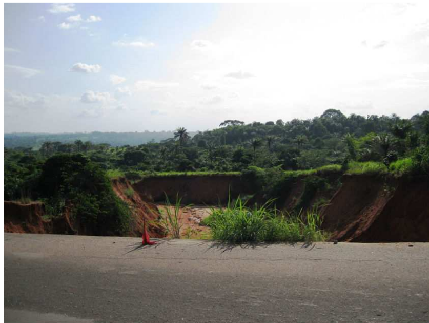
Figure 5. Gully about cutting an asphalt surfaced road
