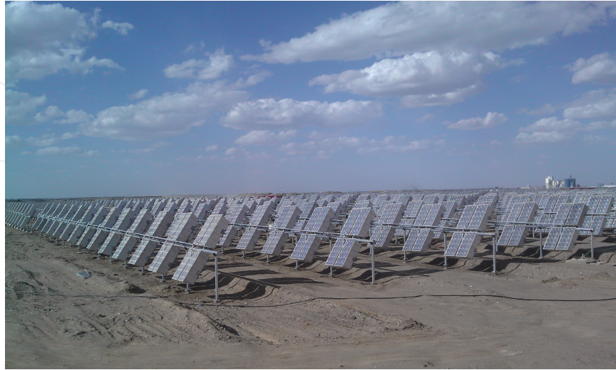
Figure 17. power plant installed at Golmud Qinghai province China.
