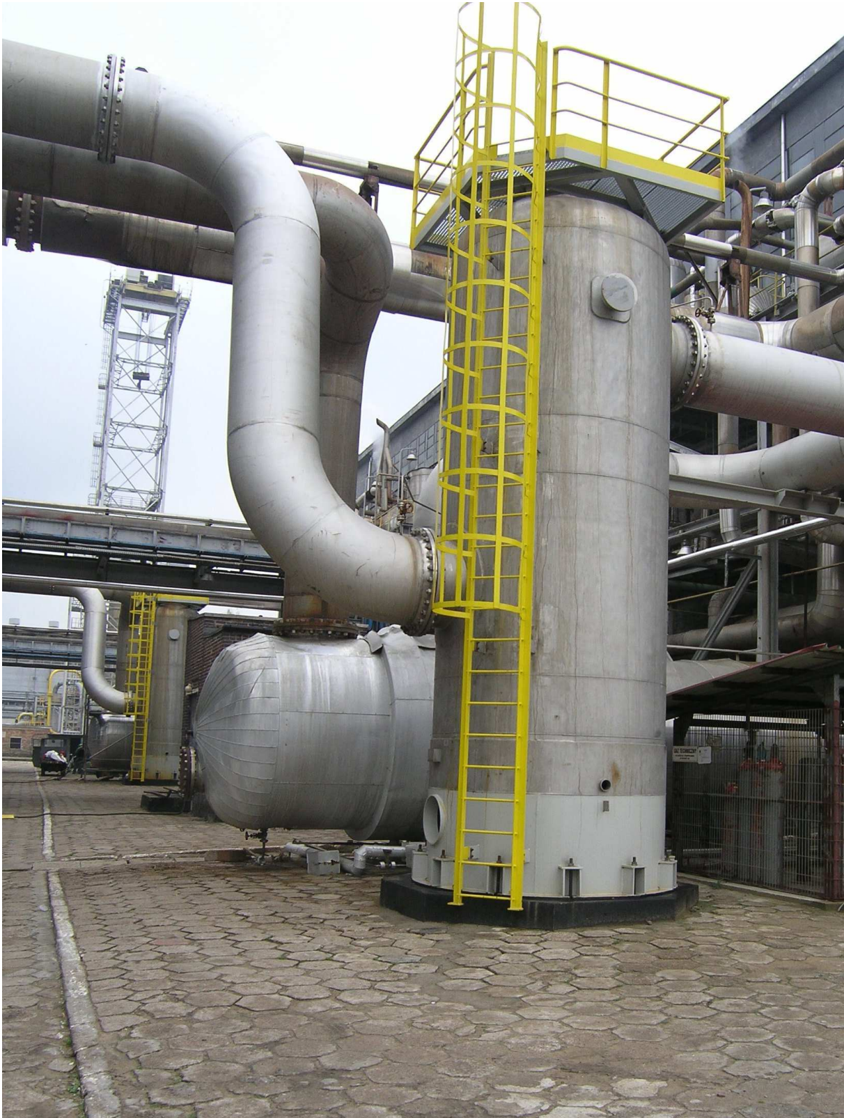
Fig. 5. Condensate separator from tail gases
