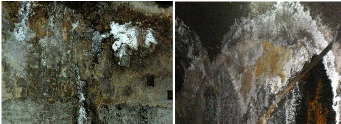
Fig. 1. Deterioration of railway tunnel (Southwestern Region, China)
