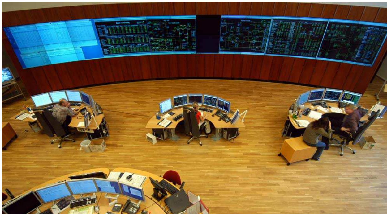
Fig. 7. Large display walls have a great impact on the control room layout.
