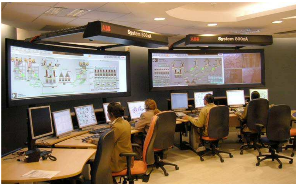
Fig. 11. Several experienced operators in a consolidated control center.
