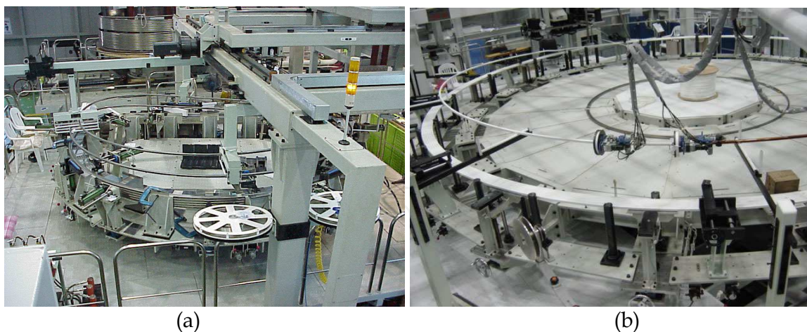
Fig. 7. The picture of coil winding stations of the TF coil (a) and PF coil (b).
