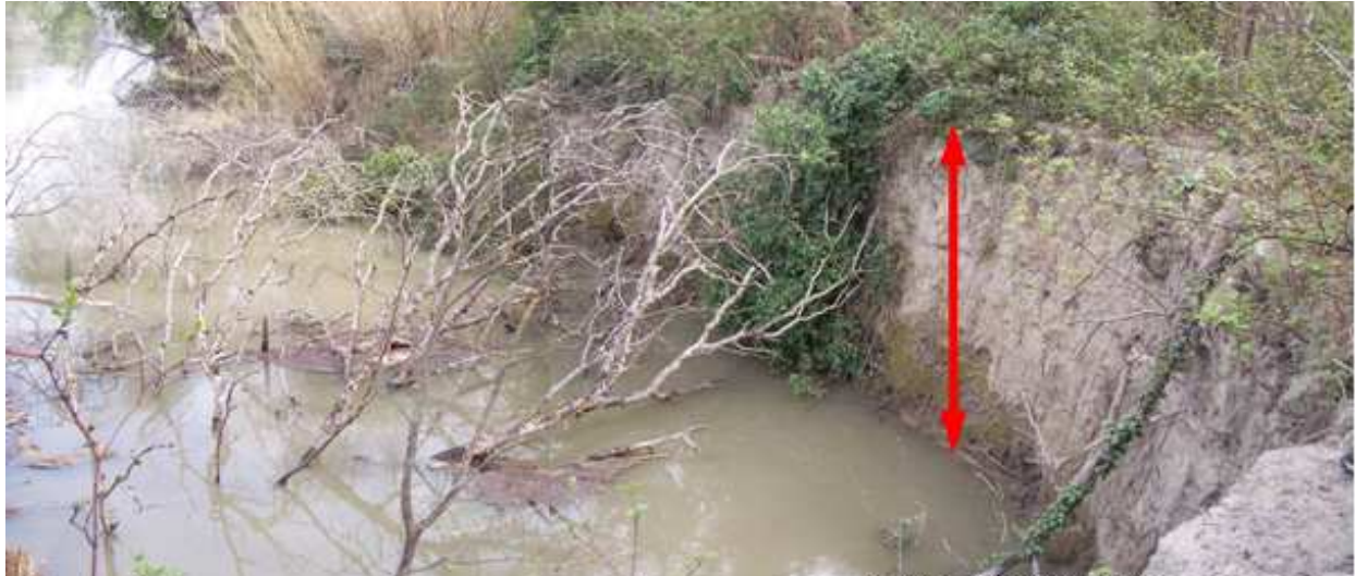
Fig. 8. Bank erosion. The red arrow represents the 3.5 m elevation gap seen on Fig. 7 (source Cemagref)
