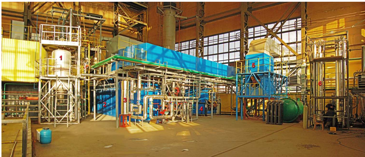
1 - The synthesis gas generator by partial gas oxidation with syngas cooler, 2 - gas turbine, 3- soot filter, 4 - water heating boiler, 5 - water cooling tower, 6 - block of methanol synthesis.
