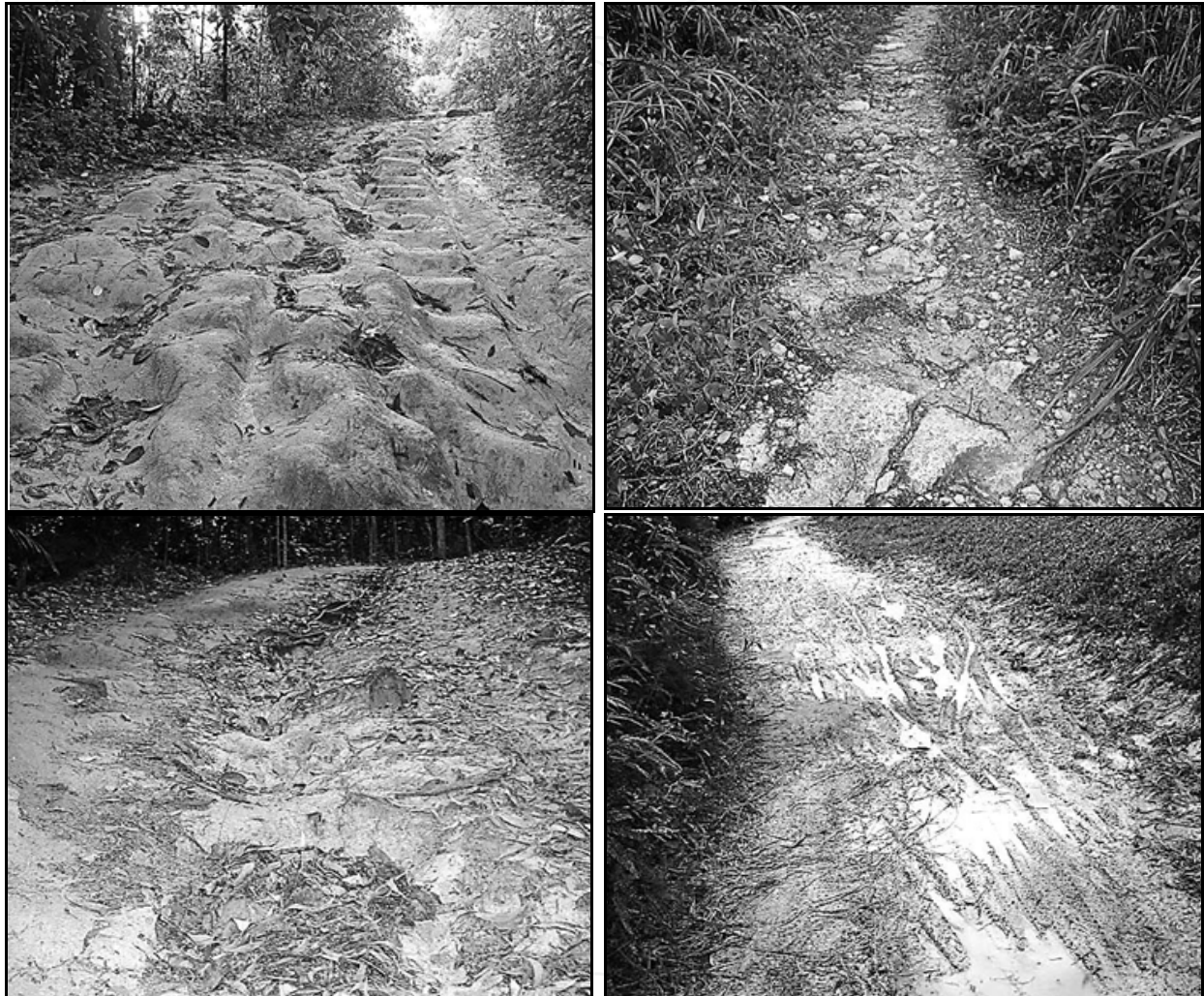
Fig. 11. Surface degradation along trails
