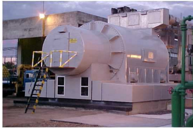
Fig. 3. Synchronous Compensator 01 of the substation Vila do Conde.
