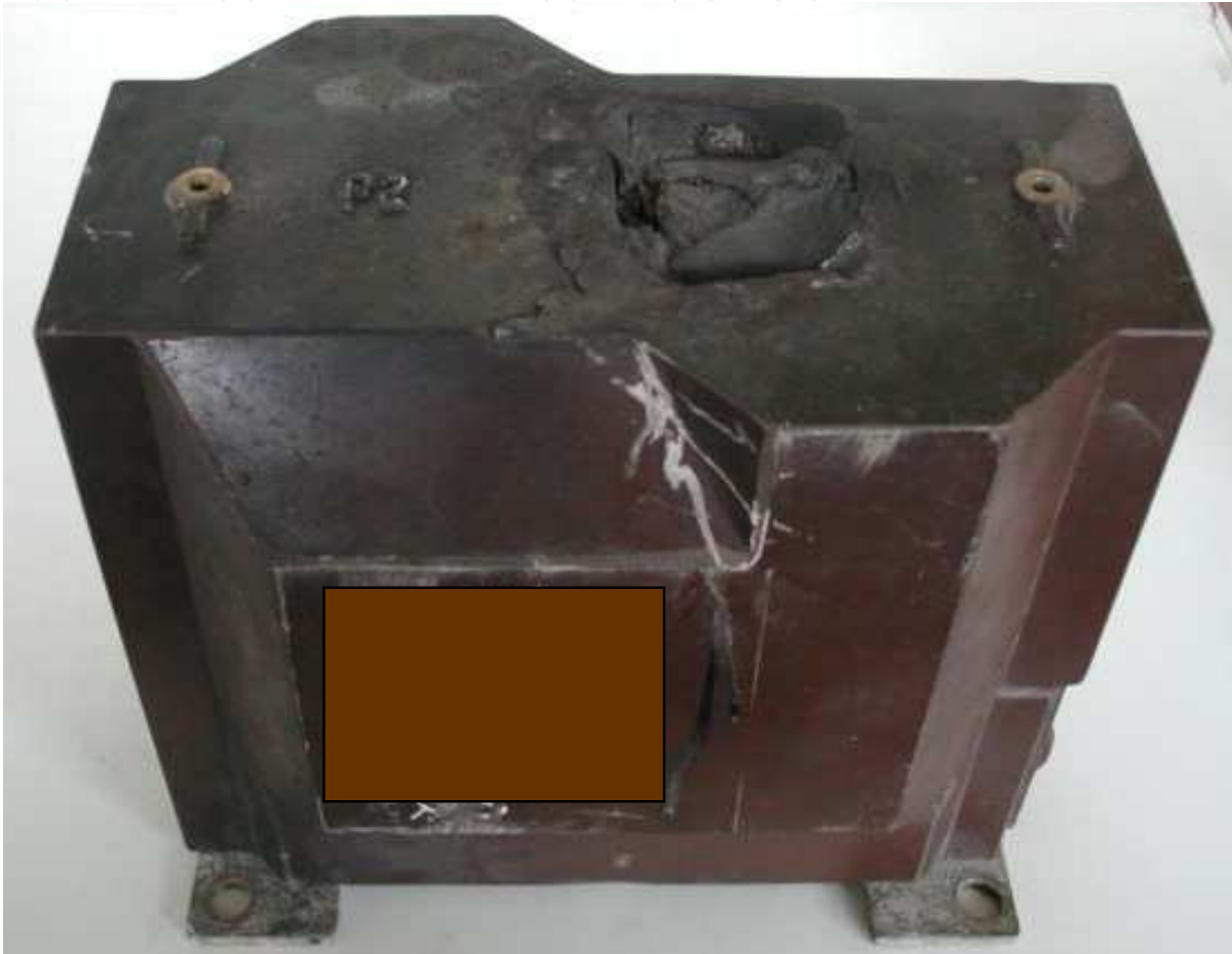
Fig. 4.3.2.1. Potential transformer that caused the failure in switchgear.
