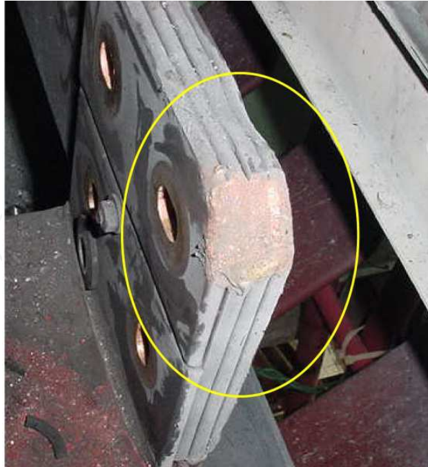
Fig. 3.5.2.1. Electroerosion damages by repetitive or intermittent ground fault arc flash.
