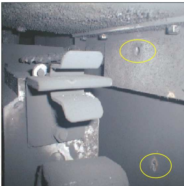
Fig. 3.5.2.2. Arc flash evidences between CT's and metallic walls.
