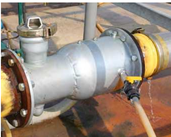
(a) Backflow prevention valve, chemical diffuser, and hose from injection pump
