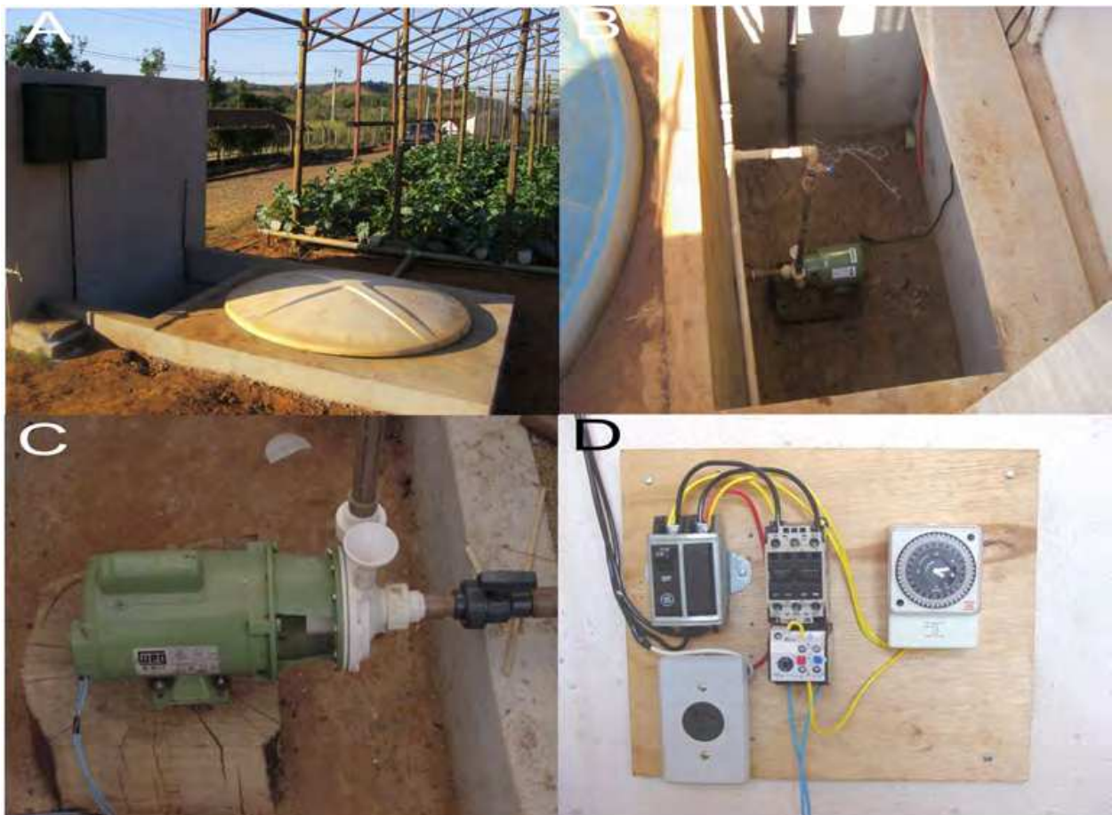
Fig. 2. Detail of the pump house (under construction) illustrating: A) Hydroponics being built by focusing the detail of water tank buried in the soil to avoid heating, B) and C) Set motor pump installed in a primed (below the level of reservoir), D) Panel containing outlet, timer relay and nutritious species. Photos: IFMG Bambuí, Professor Ricardo M. Corrêa.
