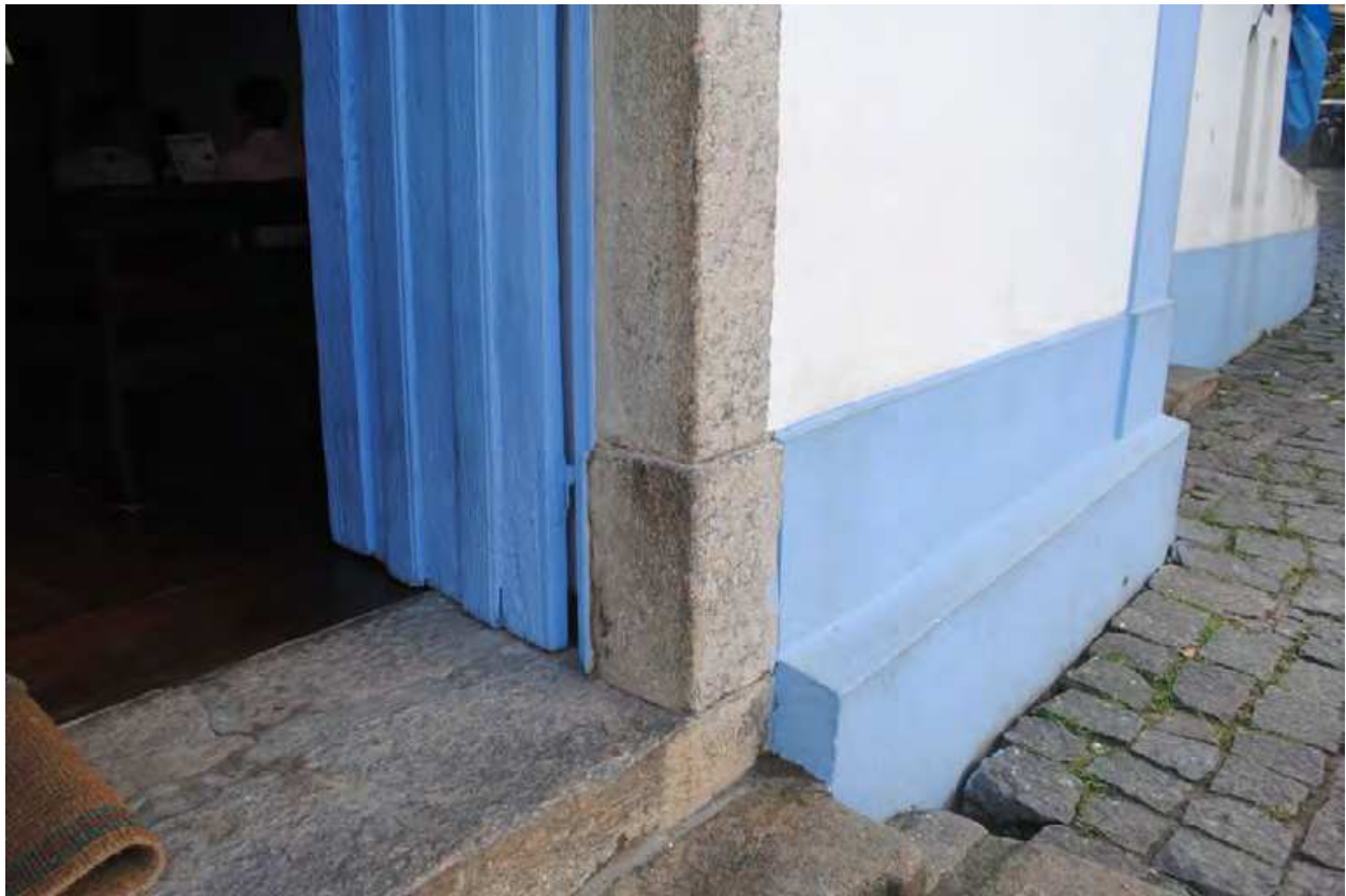
Fig. 9. Detail of a doorframe constructed in the 17th century in Rio de Janeiro.
