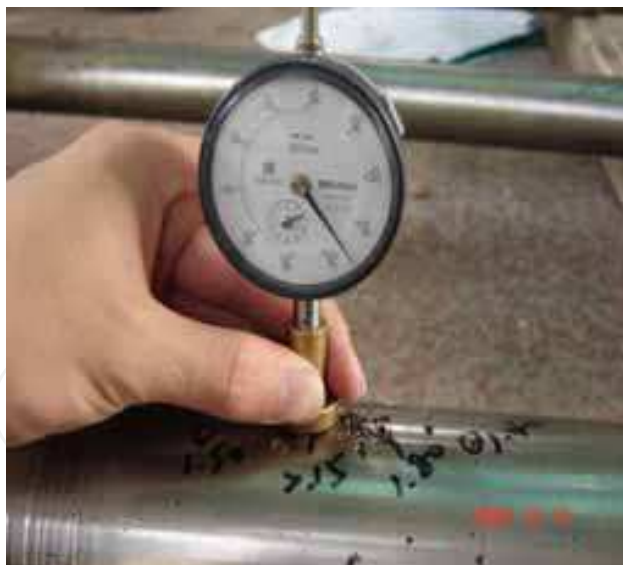
Fig. 2. Measuring depth of pitting deep
