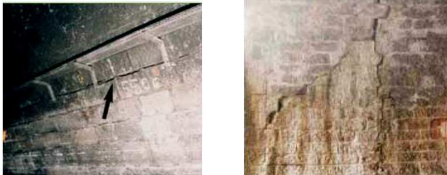
Fig. 9. Illustration and examples of degradations of masonry tunnels.
