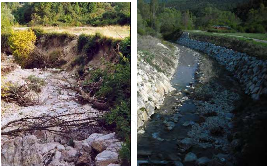
Fig. 9. The Céans river bed in 2004 (left) and in 2011 (right) (Southern French Alps). The bed of the Céans was entrenching strongly in the last decades, due to a great decrease of erosion and sediment transport. The river banks were falling regularly in the entrenched bed (left), obliging the authorities in building new embankments to protect surrounding areas from destruction (right).
