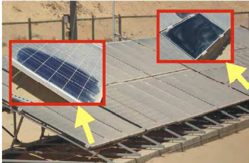
Fig. 4. Dust layer accumulation on PV modules in Egypt (Ibrahim et al., 2009).
