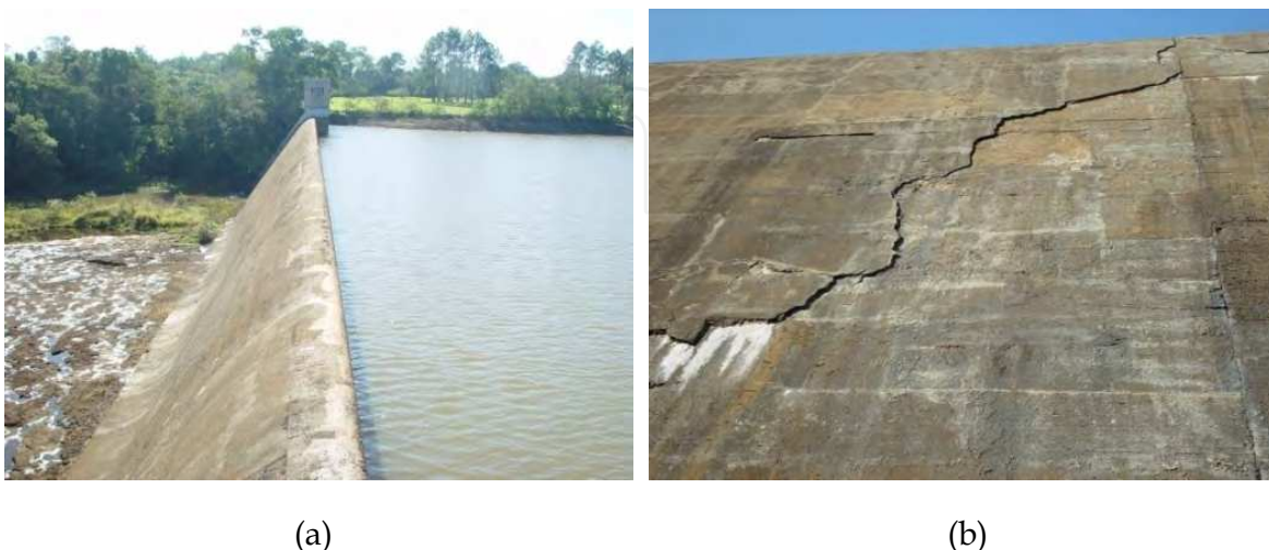
Fig. 8. (a) Overview of the spillway of the dam. (b) Detail of the displacement of the surface caused by hydraulic abrasive processes.
