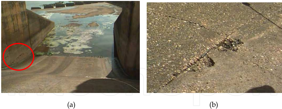
Fig. 2. (a) Spillway dam presented deterioration by abrasion. (b) Defects in the concrete structure caused by abrasive process
