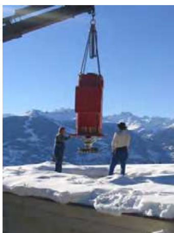
Photo 1. La Zour: the setting of the runner and the generator.
