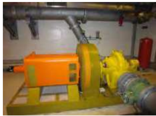
Photo 26. Reverse pump set on the treated wastewater (case study Nyon).
