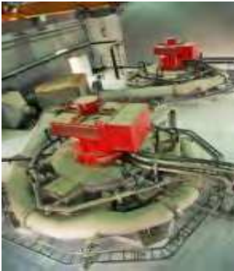
Photo 13. Two 5 nozzle Pelton turbines set on the raw wastewaters of Amman City, As Samra plants (Jordan) ( H = 104 m, Q = 2 \times 1.25 m 3 /s, P = 2 \times 830 kW, E = 12.5 GWh/year, 2007).
