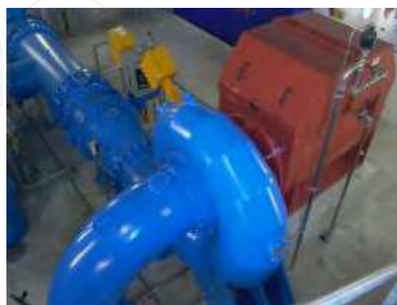
Photo 18. Aire-La-Ville: the Francis turbine set on the attraction discharge, close to the fish pass entrance.
