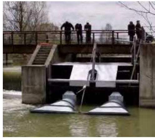
Photo 4. Marchfeldkanal: the turbines.
