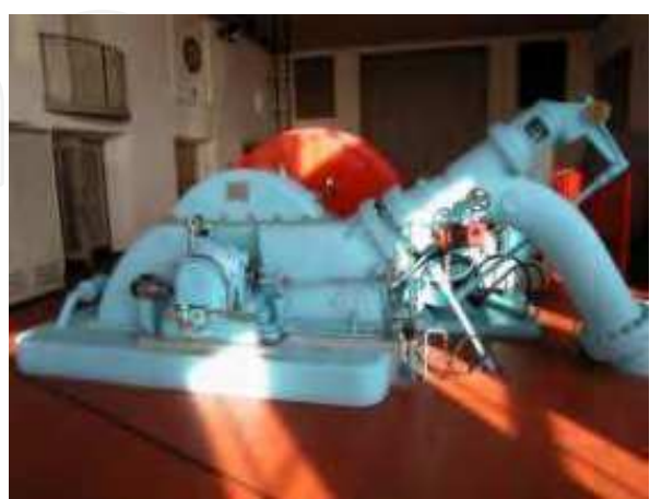
Photo 2. Mülhau: Drinking water turbine (2-nozzle Pelton turbine).
