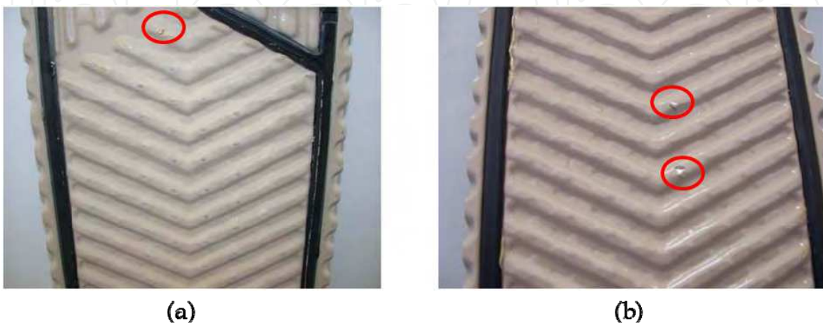
Fig. 14. Coated heat exchanger plates from heating section: (a) A2 coating, (b) A10 coating.
