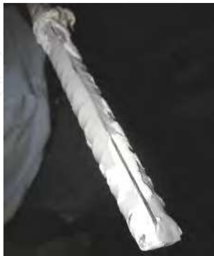
Fig. 19. Interlocking surface in an anchor installed into a hole which is not filled with epoxy (Photo by Dr. Halil Nohutcu)
