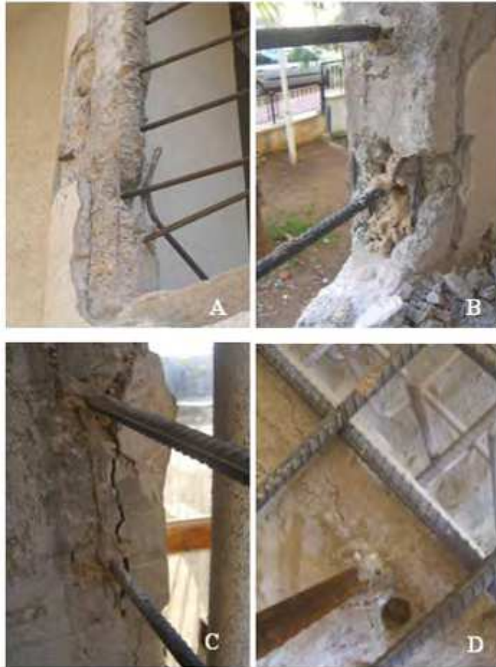
Fig. 18. Poorly implemented anchor examples (A, B: anchors implemented on defective surfaces; C: Anchor implemented near a crack; D: Anchor fracturing the concrete during the tensile test)
