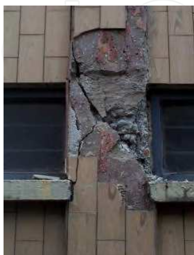
Fig. 8. shear failures in columns (California 1994)
