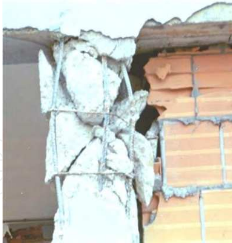
Fig. 9. Shear failure of column (Italia 2002)
