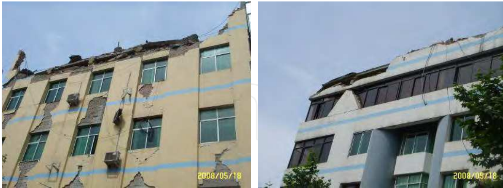
Fig. 4. Failure of the parapet wall
