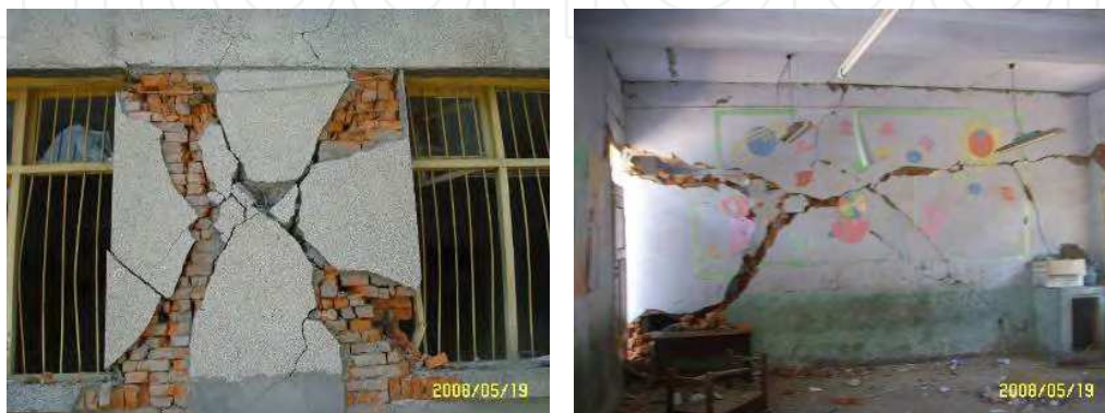
Fig. 8. Through cracks on the longitudinal and transverse load-bearing wall
