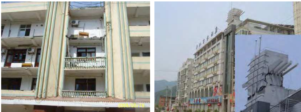
Fig. 5. Falling of the corridor fence and horizontal crack of the protruding member
