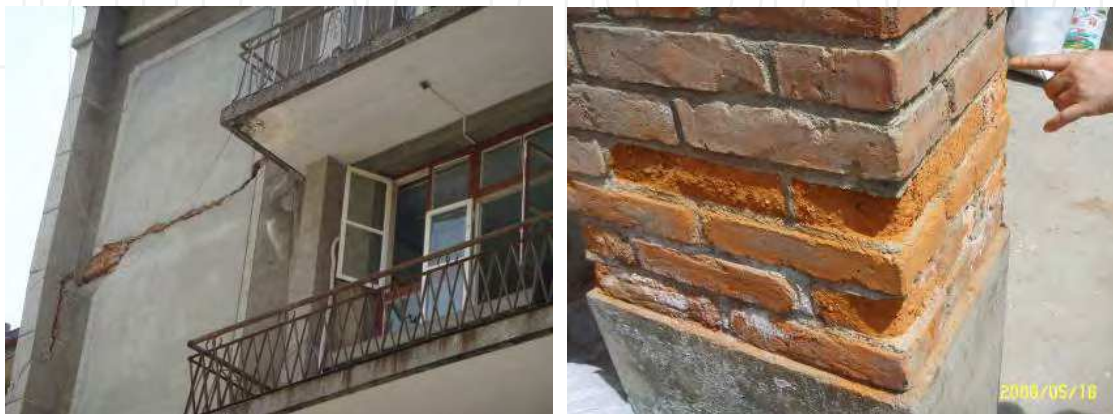
Fig. 2. Horizontal cracks on the wall or the bearing brick column
