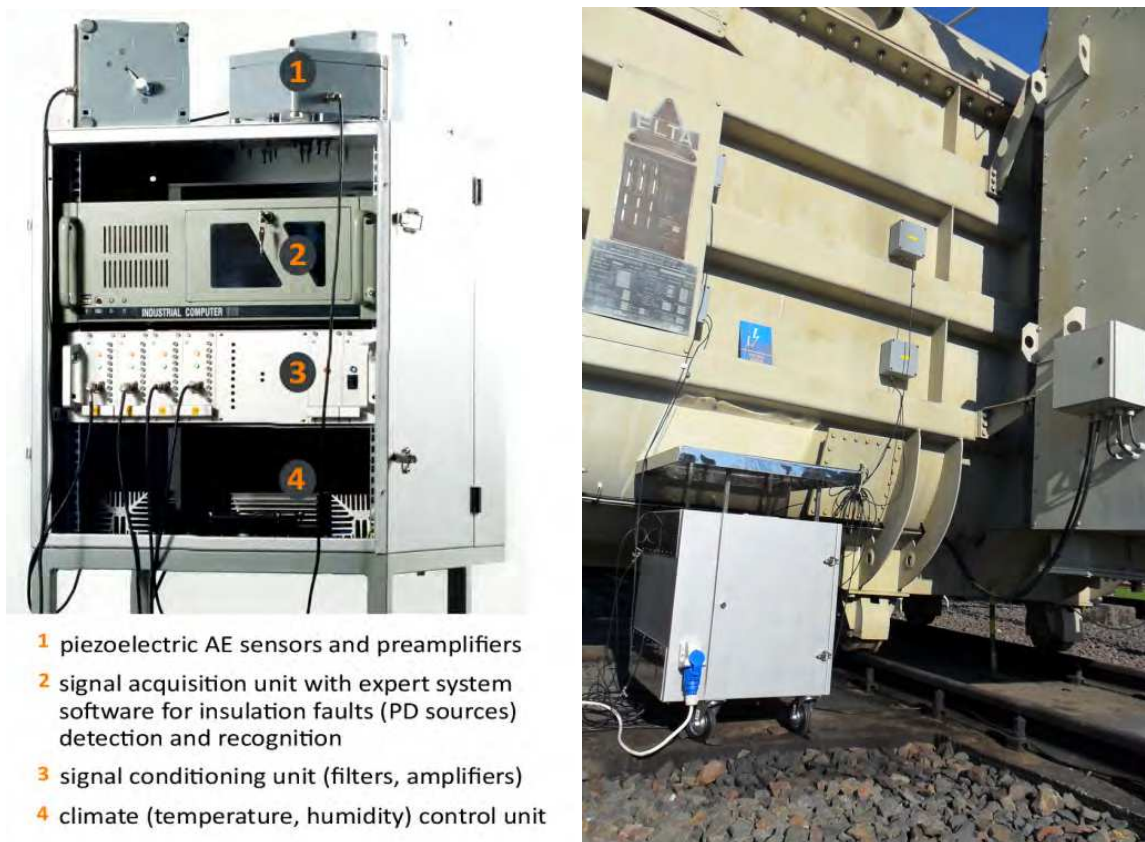
Fig. 1. System for large power transformer on-line monitoring based on AE method
