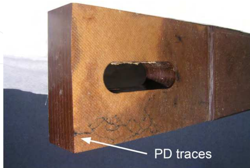
Fig. 23. The location of embedded metal particle under the surface of pressboard beam of S/P switch (the PD tracking originated from this area).
