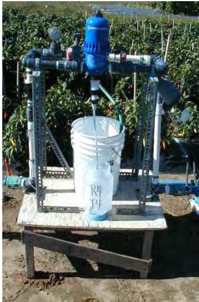
Fig. 5. A Dosatron ® injection pump injecting a pesticide in bell pepper, Bridgeton, NJ.
