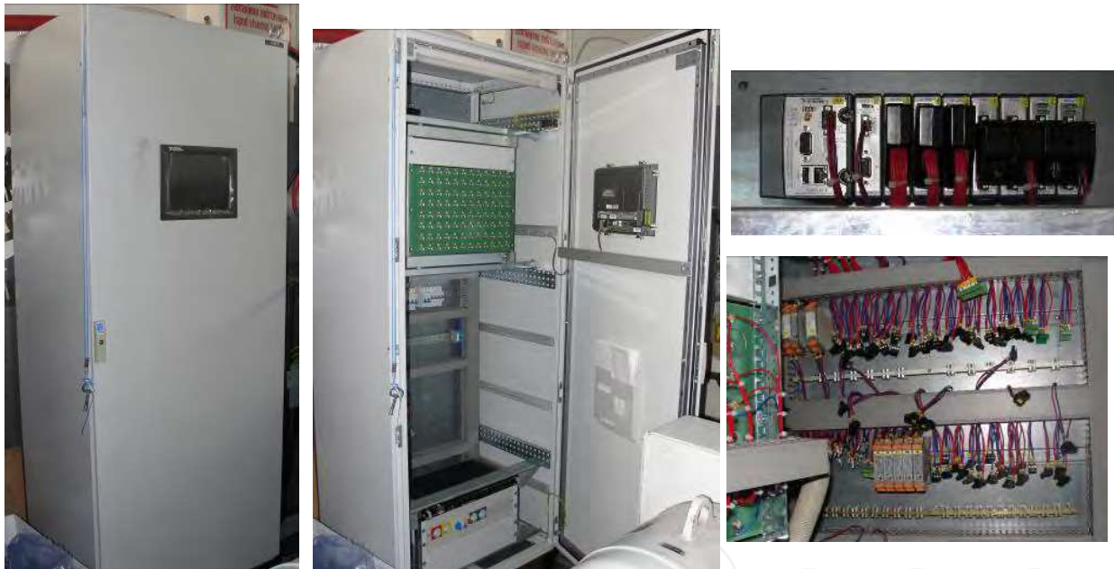
Fig. 13. Measurement cabinet for measurement systems installed on all three generators in hydro power plant Vinodol
