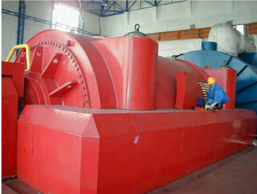
Fig. 14. Turbo-generator 250 MVA in Plomin 2 thermo power plant
