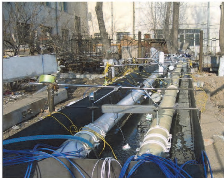
Fig. 37. Instrumented PVC pipe in water tank
