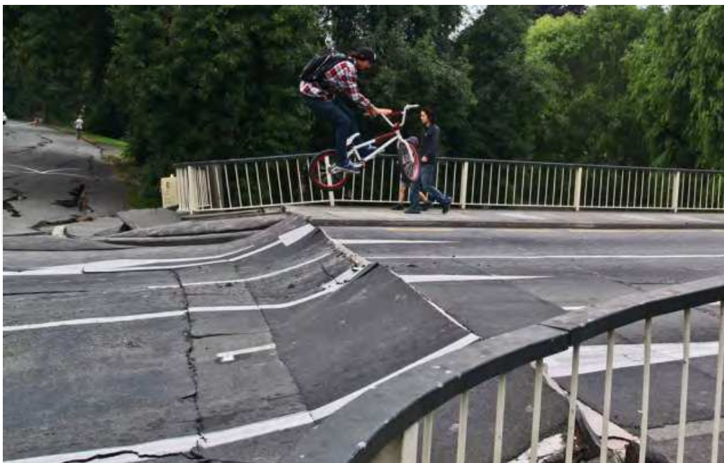
Fig. 47. Settlement of Approach Fill at Bridge Abutment Formed a Bike-Jump for a Youngster. http://otilya.com/view/News/Asia-Pacific/New-Zealand
