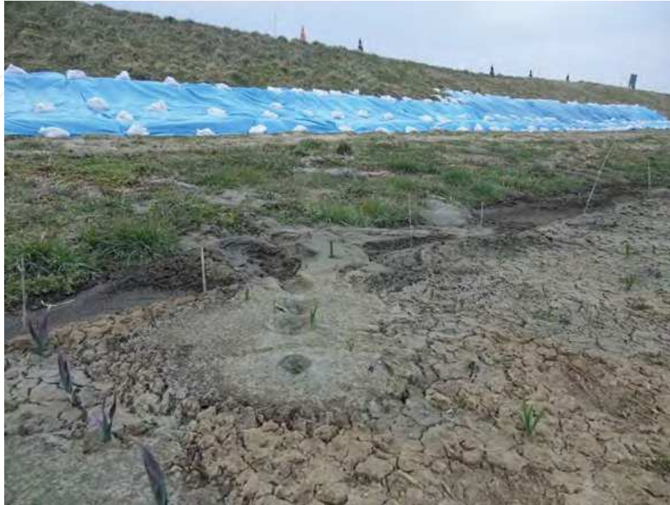
Fig. 44. Levee Slope Repair and Sand Boils at Toe, Japan. (JSCE 2011)
