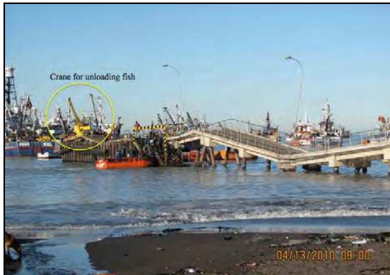
Fig. 22. Distorted Fish-Unloading Concrete Pier at Coronel Port, Chile. (TCLEE 2010)
