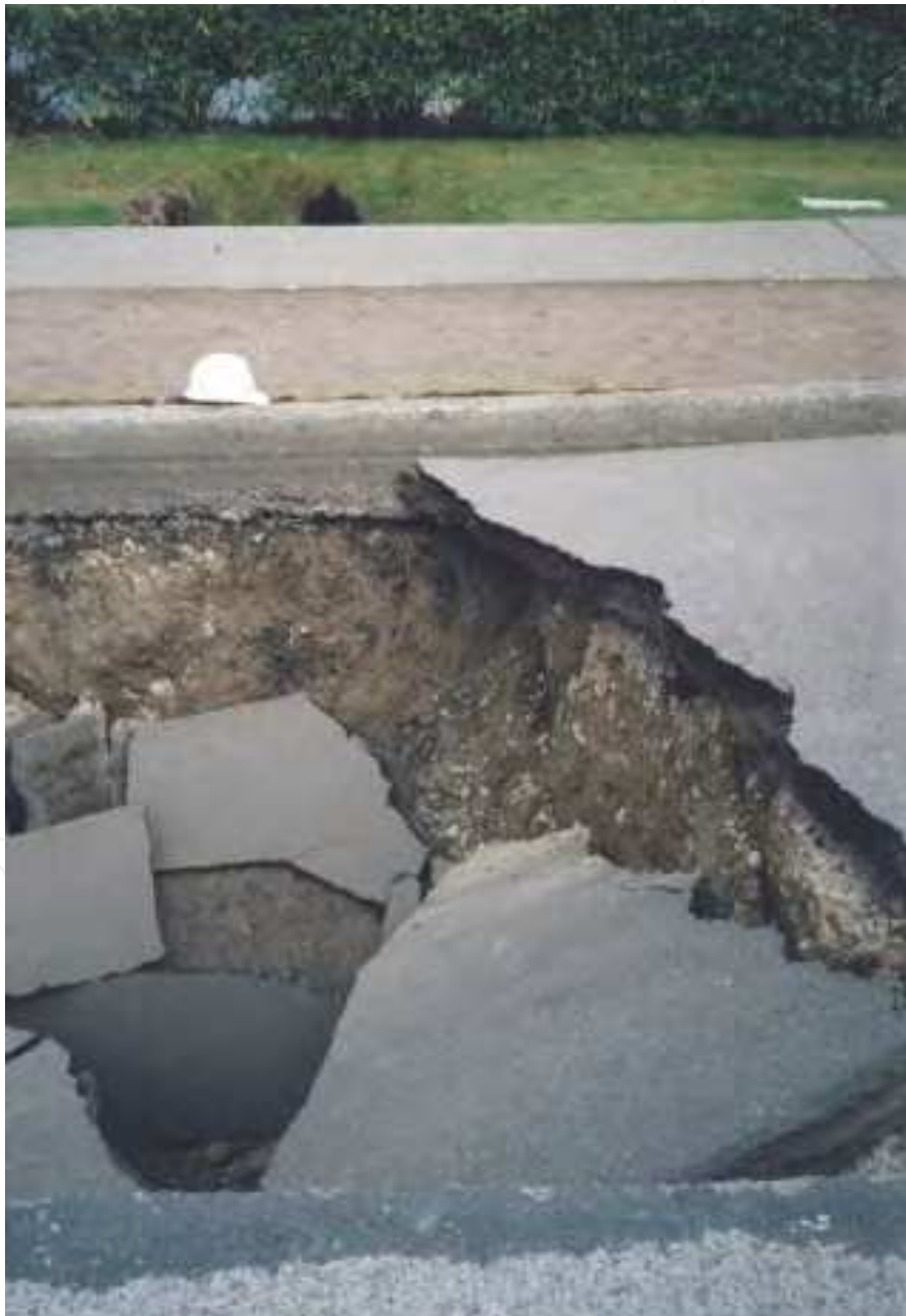
Fig. 46. Sinkhole Formed by Collapse of Roadway During Earthquake, Washington, 2001.
