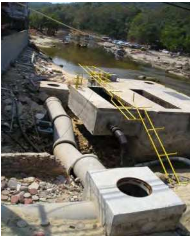
Fig. 39. Pump Station Damaged by Wave Scour, Patong Beach, Phuket Province, Thailand, 2004.
