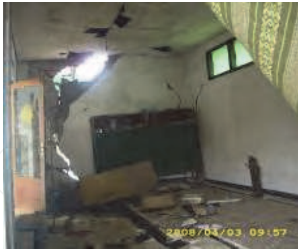
Fig. 29. A mosque located in the Renokenongo village, to the east main of the vent is damaged due to fault reactivation. At this location a lot of fractures were oriented NE-SW, and these are patterns of the Watukosek fault system.
