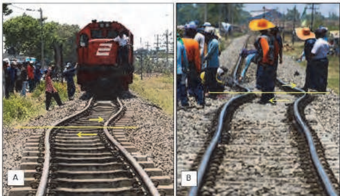
Fig. 11. Shear stress have damaged nearby infrastructures such as the dextral movements of a railway, bursting of a gas pipeline and numerous breakages of water pipelines at the same location further supports displacements along faults. (A) The railway bent to the west of main vent on September 2006. Offsets that occurred approximately 40 cm with orientation direction NW - SE. (B) At the same location, the railway was bent again in October 2009, with an offset of approximately 45 cm. The bending of the railway line is due to fault reactivation that often has differential movements which created shear stress.
