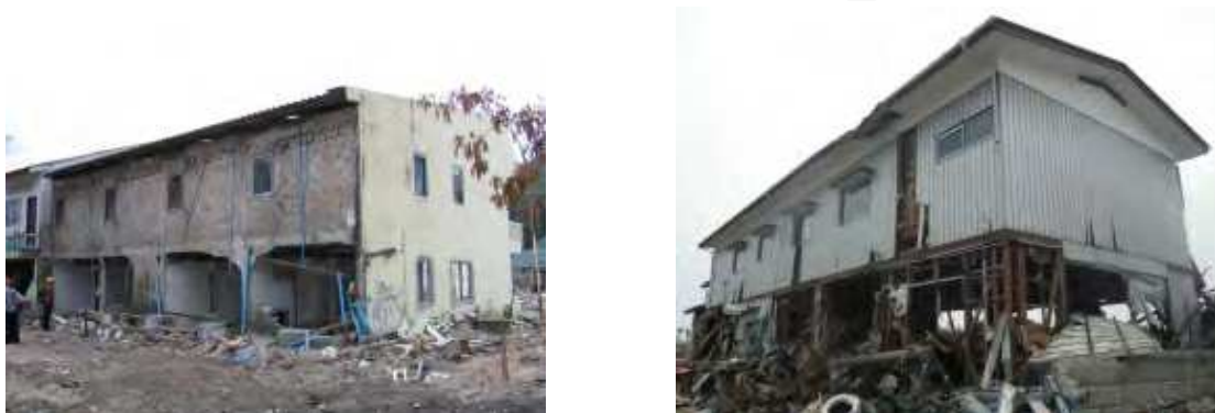
Fig. 25. Examples of building damage in the case of the 2004 Indian Ocean tsunami in Thailand and the 2011 Tohoku tsunami in Japan
