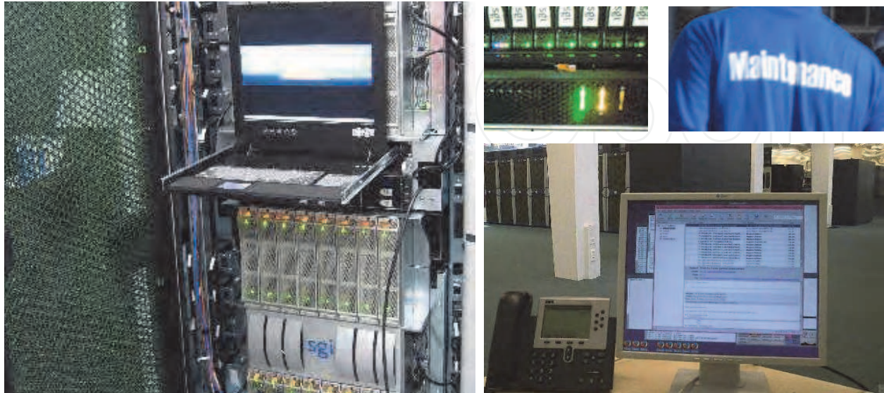
Fig. 6. Operating using local console access, remote access, monitoring and physical maintenance.
