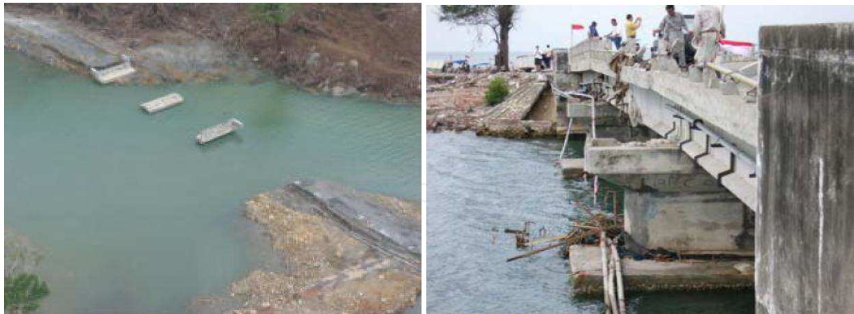
(a) Total Wash-Away of Deck (Unjoh, 2005) (b) Excessive Deck Displacement (Yim, 2005)
